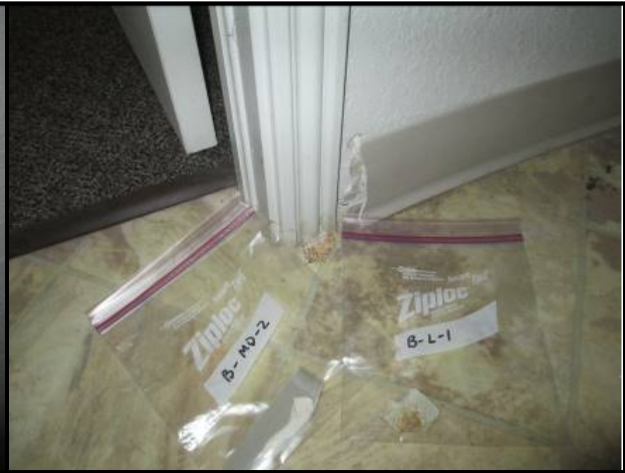
Photo 11: South Unit Linoleum and Molding
